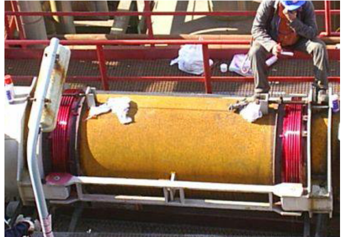
Inspection of an assembled metal expansion joint, made for FCC-plants
